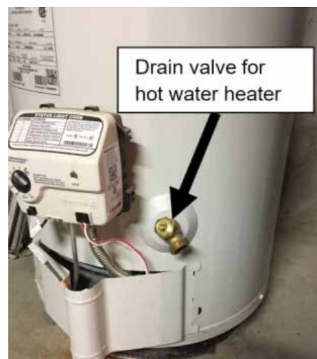
FIGURE 6 Water heater with drain valve
